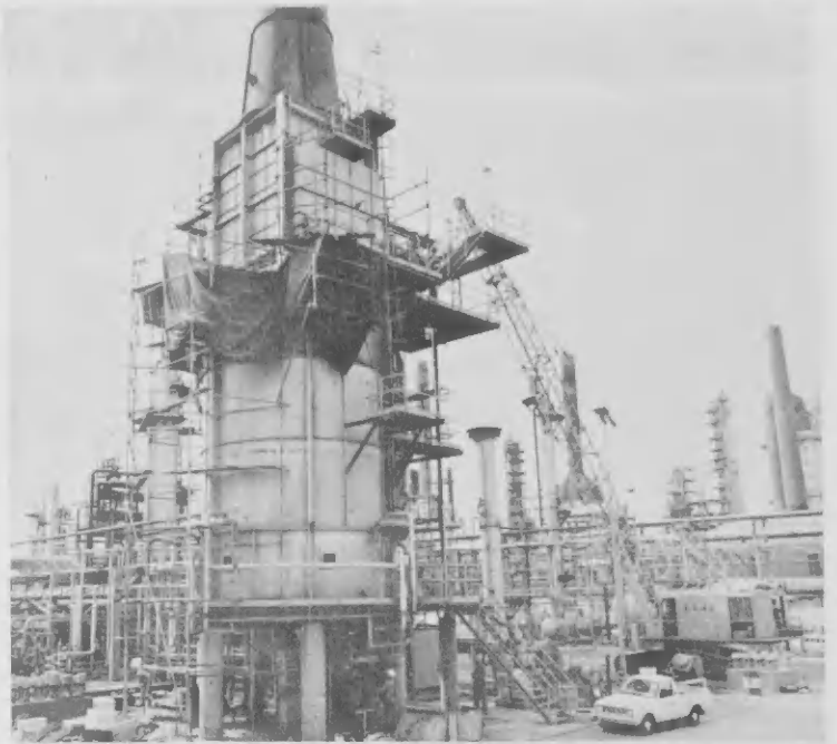
Scaffolds, tarpaulins and a nearby crane bear witness to the recent turnaround at the Kerosene Hydrofiner Unit of the HDS-I Project. Stelashi, Ionanan y un grua den vecindario ta testigo di e reciente revision general di e Kerosene Hydrofiner Unit di ■ Proyecto HDS-I.
